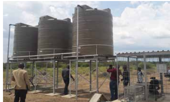
Mapanda borehole fully installed and operational in the Kavango region
