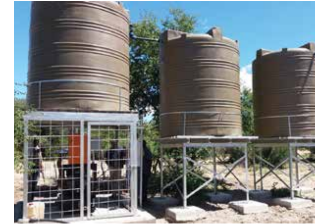
Fully equipped borehole with deasel powered monopump
