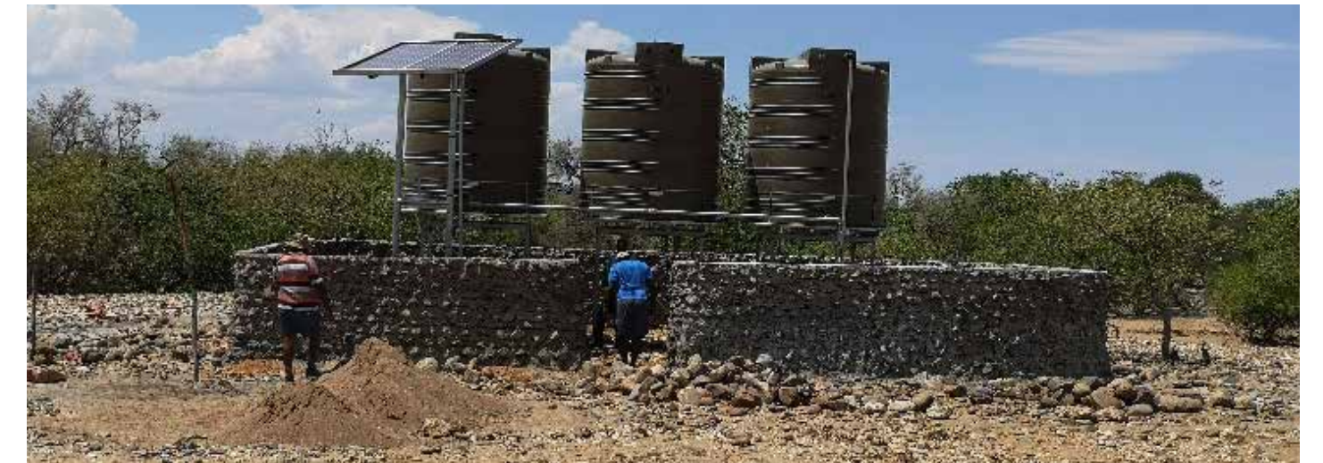
Completed solar installation in the Kunene region
